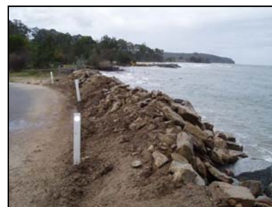
Part of the Hazardous Land at Wharf Rd
